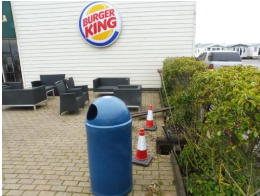
Leak location by isolation valve outside Burger King
