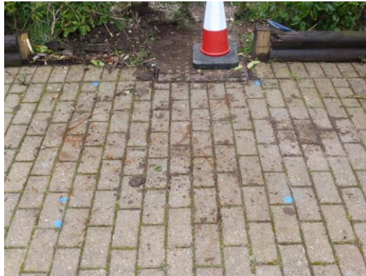
Leak location marked up
