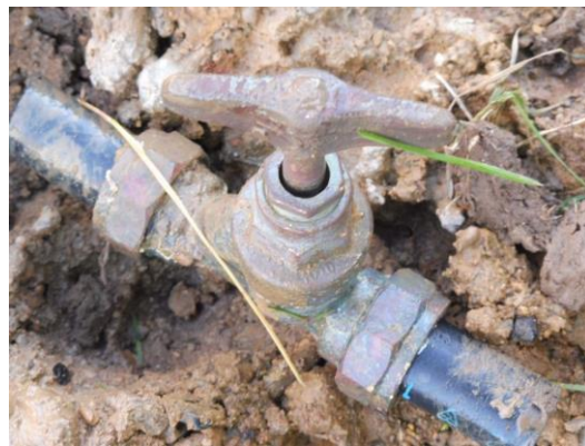
Leaking stopcock gland - 11 Spruce Bridge
