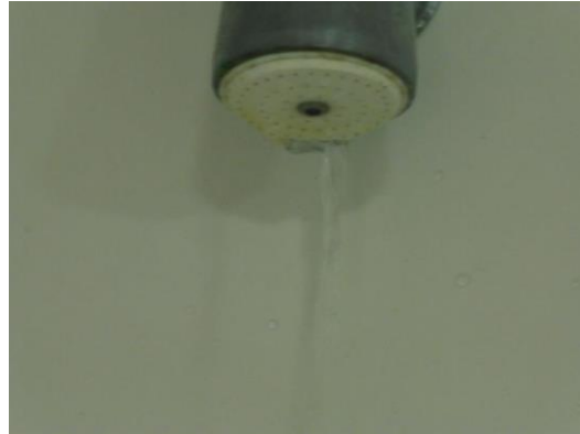
Disabled shower - Leaking shower head
