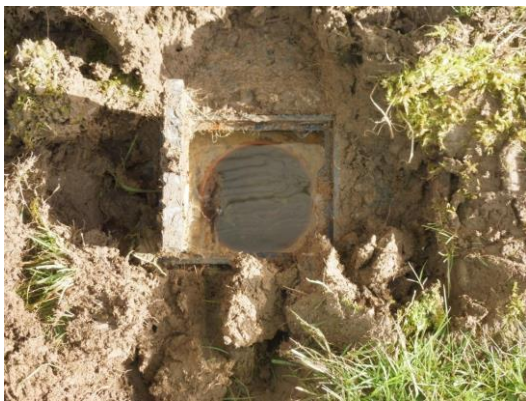
Leaking stopcock - 50 Spruce Bridge
