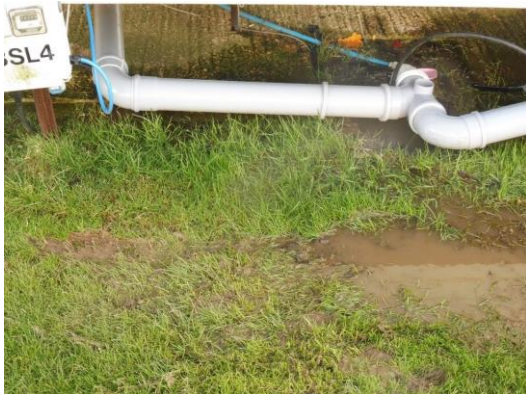
Leak at Birchtree Side L4
