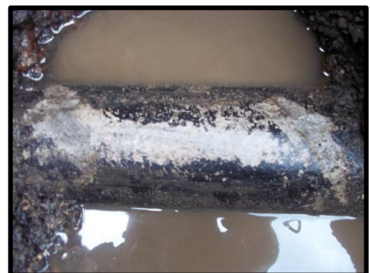
Picture 4 – Asbestos Pipe
