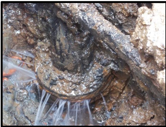
Picture 1 – Leaking Flange Joint
