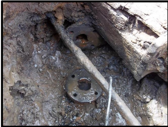
Picture 3 – Where T Joint removed with live cable
